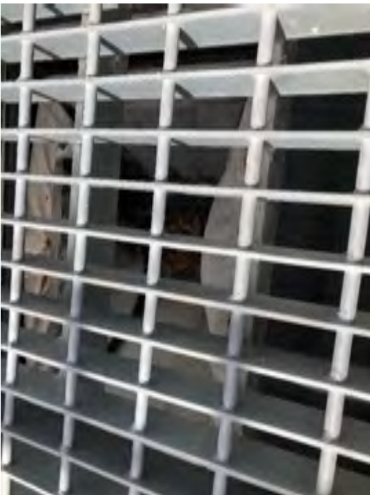
Figure 1: Stormwater Pit showing filter sock
